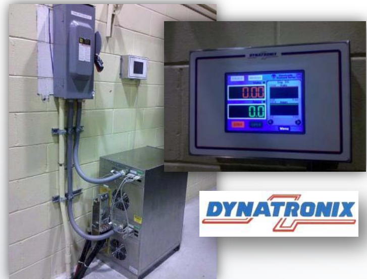
Activation Tank Power Supply
